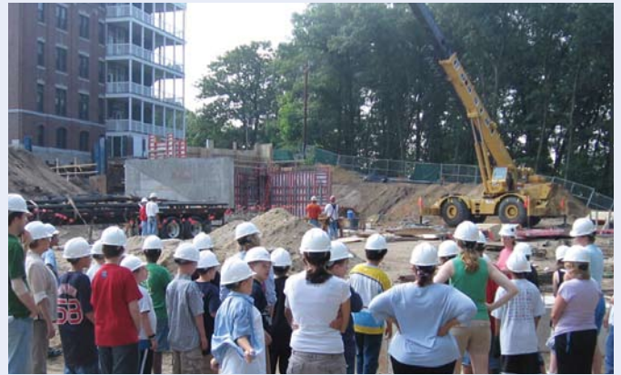
Students, residents, and staff get a first-hand view and tour of the construction of the new Adolescent Center courtesy of Barr & Barr Builders Project Superintendent K. C. Lavery and Project Manager Marcia Carlson.
